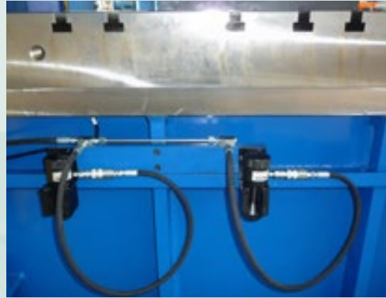
Pull cylinders on bolster with parking stations
