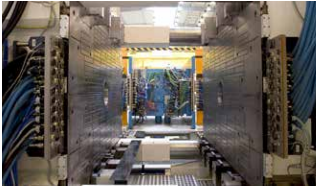
This 2700 t injection molding machines with horizontal loading, has standardized multi couplers on the movable and fixed side of the machines. Connections for cooling water, hydraulics for core pull cylinders and electric for heating and signals, are automatically connected and disconnected. This connection takes less then 30 seconds. All couplers feature the leak proof couplers, keeping floor and envirement clean.
