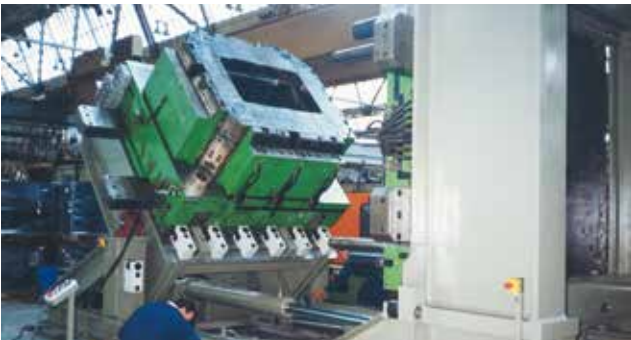
For a well known German manufacturer of plastic containers EAS equipped several large injection molding machines up to 6000 t with an adaptive hydraulic clamping systems, an air cushion mold change car, several mold storage racks and an inspection unit for molds up to 100 t.
